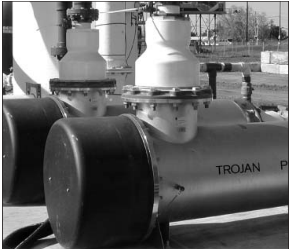
The Trojan UV-oxidation system at Stockton.
