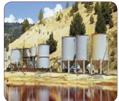
The biphasic lime system treats an AMD volume of 3.5 million gallons each summer before releasing it to Leviathan Creek.
